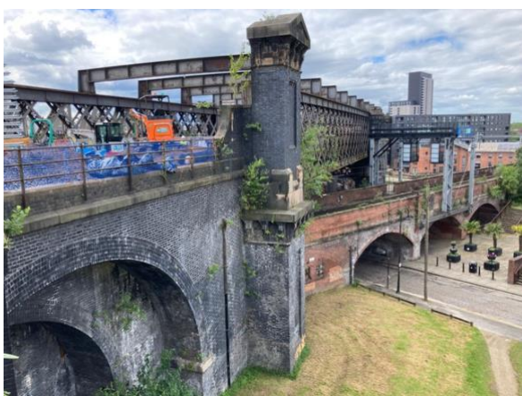
Viaduct showing construction equipment engaged in developing the Sky Park along the rail track.
